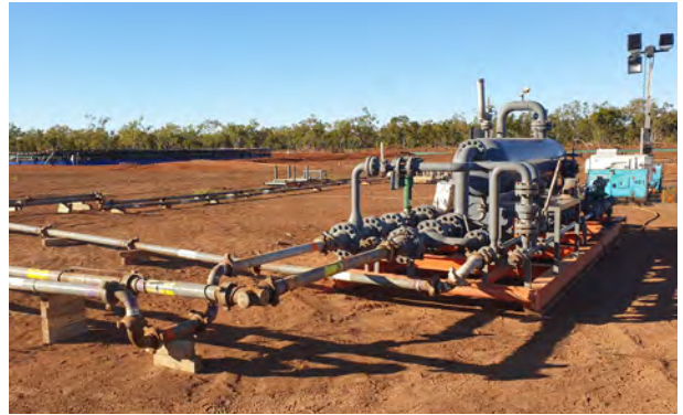
Image: Separator on Carpentaria site
