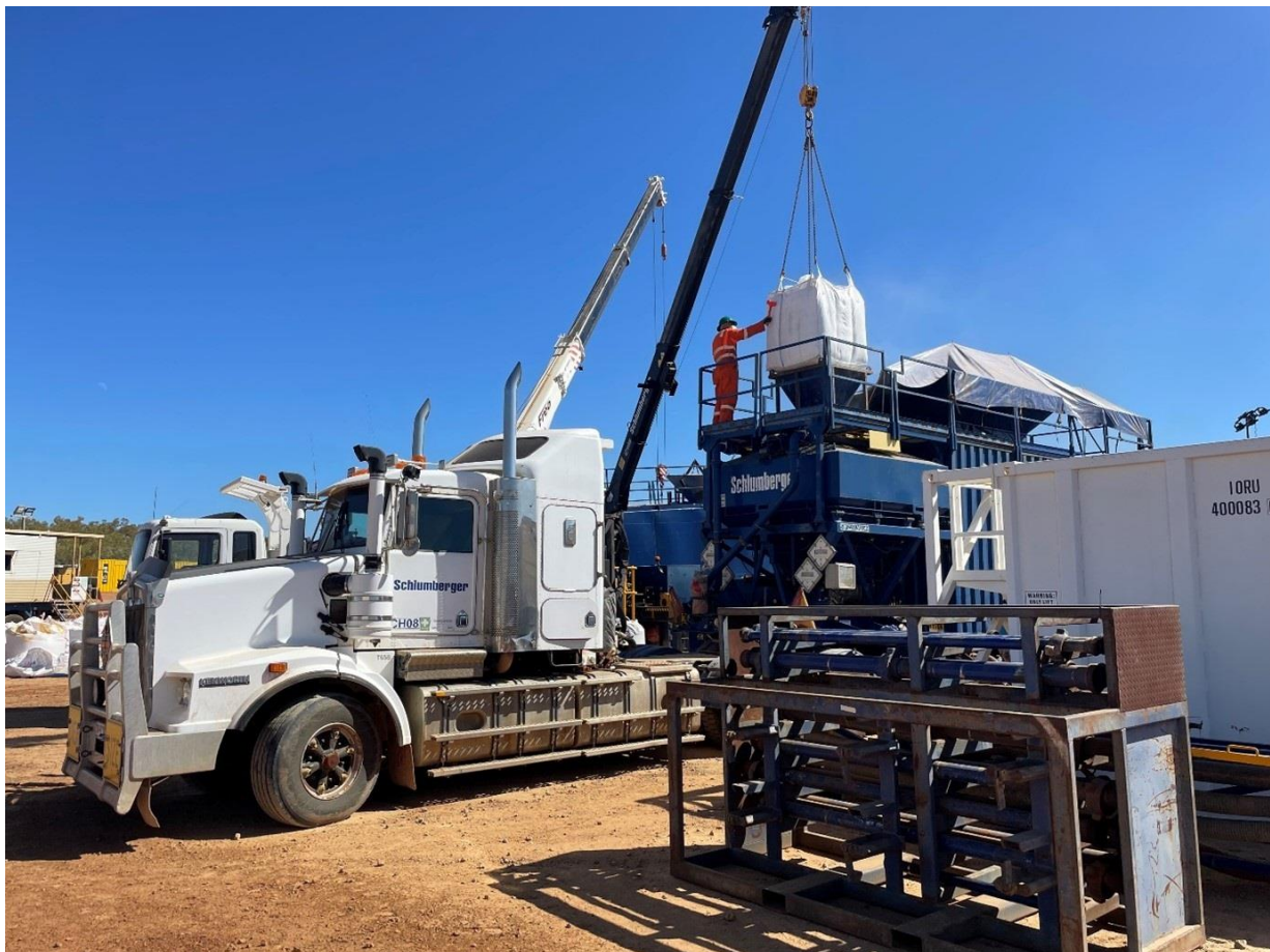
Loading proppant sand into the sand blender in preparation for a hydraulic stimulation
